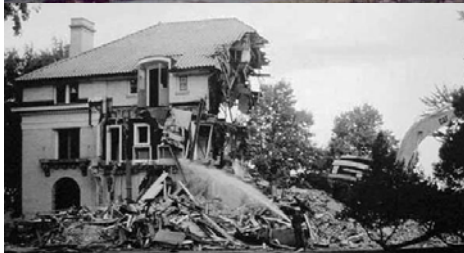
Before and After. This landmark house in Elkhart, IN, was purchased by new owners for its prominent waterfront site, and subsequently demolished, with neighbors caught off guard.
